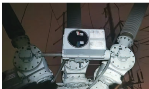
图2 故障户外PASS开关设备
